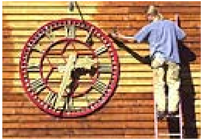
Paint: Paris Hamilton of Ely, applies a fresh coat of wood stain to the wall behind a decorative clock on the side of the Piragis building in Ely, Minn., Wednesday afternoon, Sept. 29, 2004. Wednesday's sunny skies and mid-60 degree temperatures drew people outside to try and finish up their summer and fall projects before wet, cold weather arrives on Friday. (AP Photo/Mesabi Daily News, Mark Sauer)
